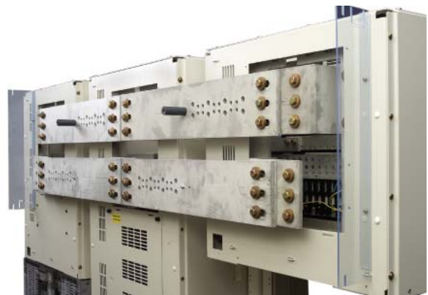
Copper Inter-bay Bus Bars (shown with cover removed for detail)
