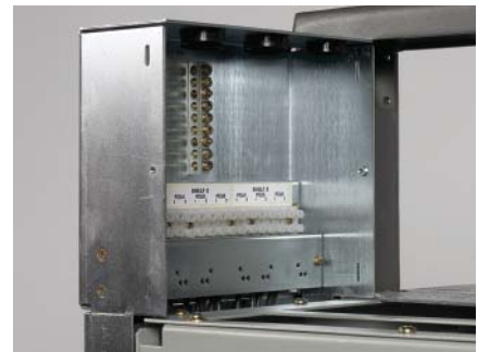
Top AC Wireway Input (cover removed)
