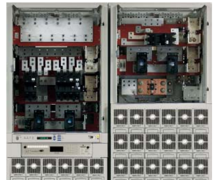
Modular Distribution Cabinets
