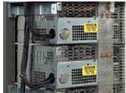
Bottom AC Wireway Input (cover removed)
