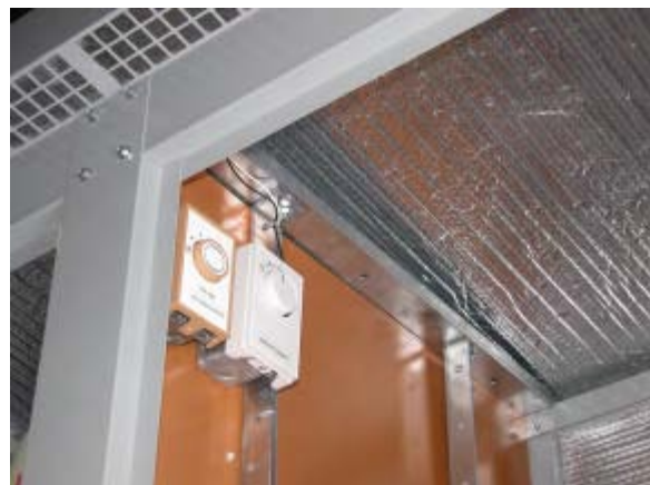
environmental options controls (heating thermostat / cooling fan control)
